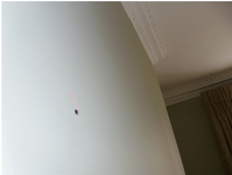
Bedroom – drilled hole to wall
