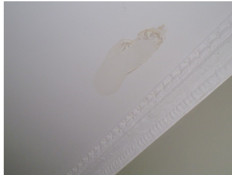
Bedroom – damp patch to ceiling
