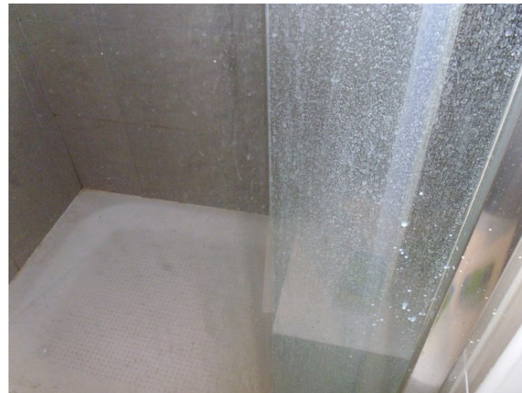
Bathroom – heaily water marked shower screen
