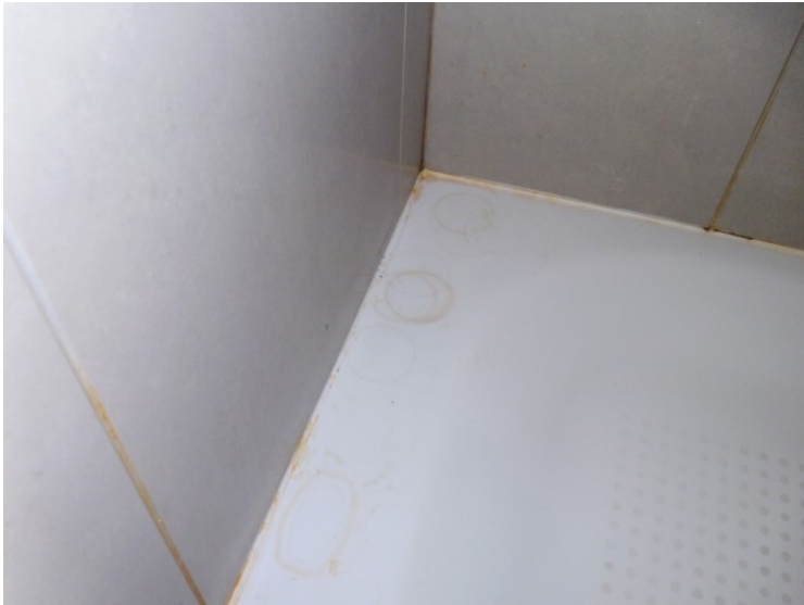
Bathroom – ring marks to shower tray
